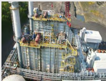
Heat Recovery Steam Generators (HRSGs)
